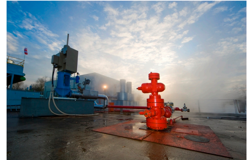
Figure 1. Landau 3-MW geothermal power station in der Pfalz, Germany. The blue pump brings the hot water up and the red one puts it back into the ground. Photo © Geox.
