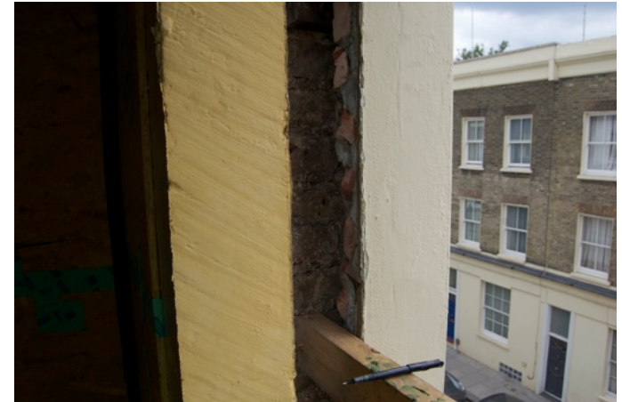
Figure 1. Internal solid wall insulation in a London home being enhanced as part of Retrofit for the Future.
